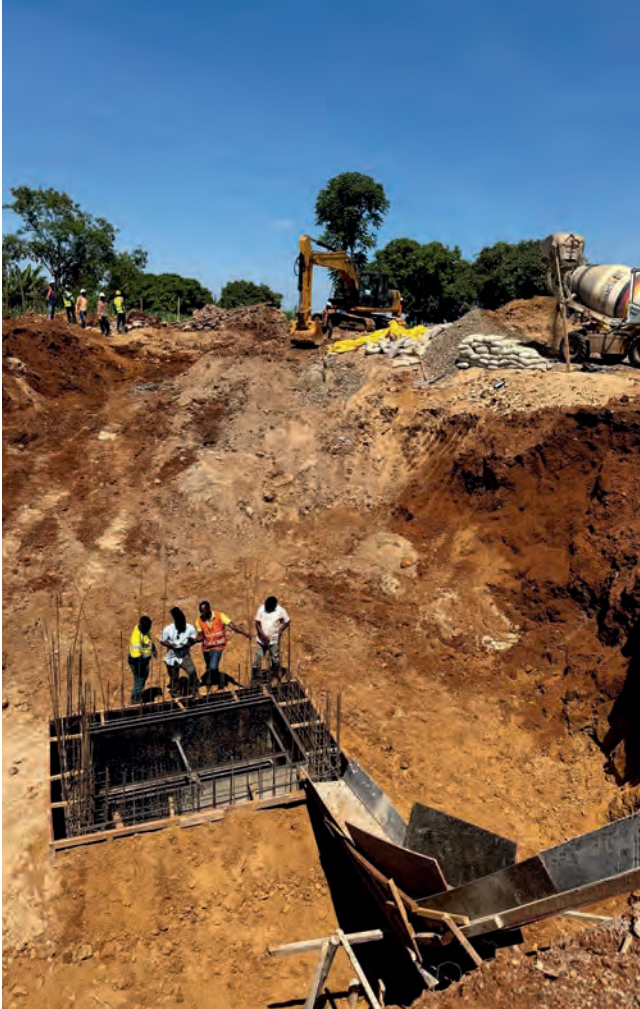
» Bahebe (blue shirt) discusses construction updates to Mwamba's Miti Minane underground mine in Geita, Tanzania.
